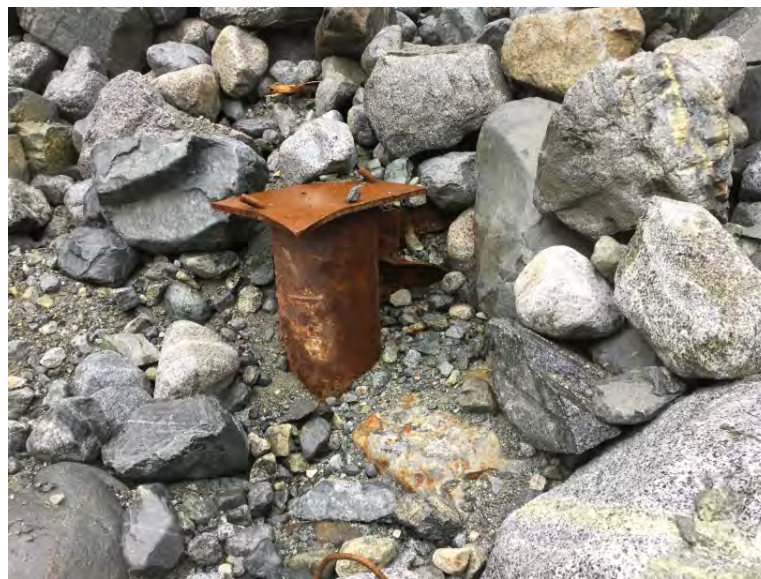
Old pipe columns still buried in approach material
